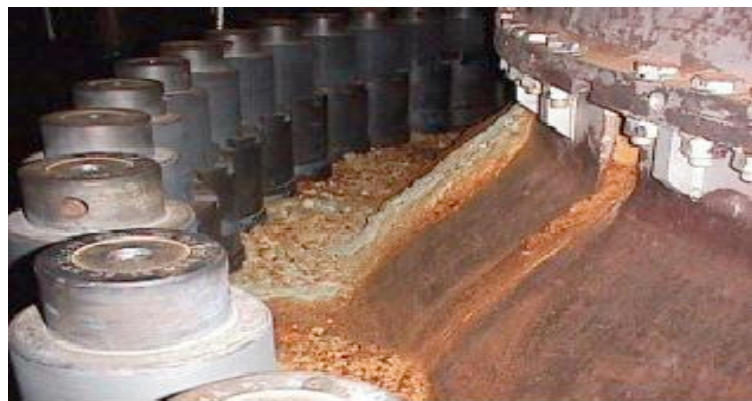
Rust-laced boric acid 'river' flowing through inspection ports on the reactor head and down onto the reactor flange during the refueling outage in 2000.
