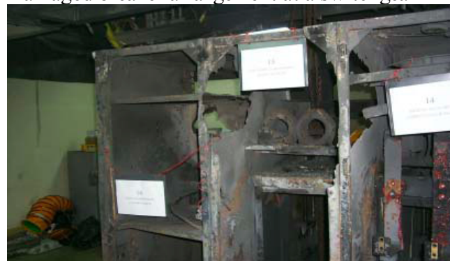
Damaged breaker arrangement at a switchgear
