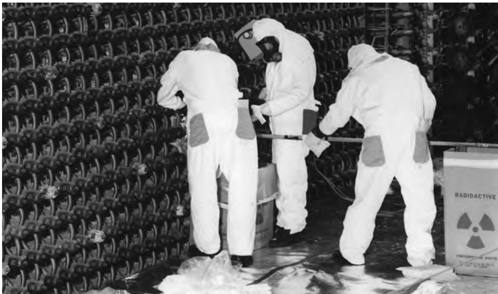
Figure 7.2. Workers taking graphite samples from the Hanford C reactor in 1994, in an early effort to test a nuclear archaeology technique. A full-scale exercise was later carried out in a British Magnox
