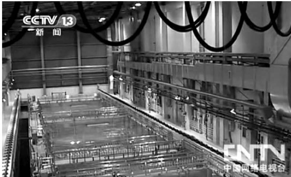
Figure 7. A cooling pond at China’s pilot reprocessing plant. The plant has the capacity of processing 50–60 tons of spent fuel per year and began operating in 2011. The hot testing of the plant in 2010
